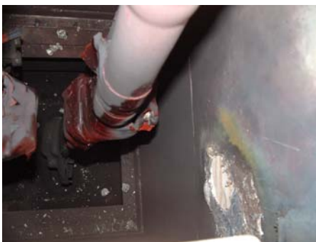
Termination Failure to Duct Wall; Cable Bus Design
